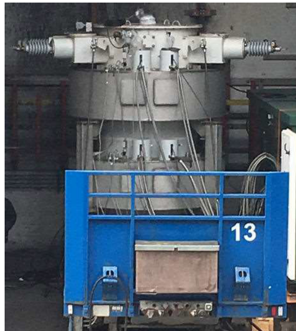
SFCL in IPH test vault, the coils are visible around the reactor tank
